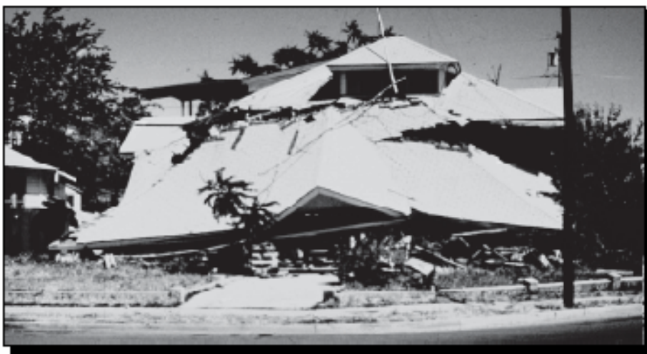
Additional damage from aftershocks
